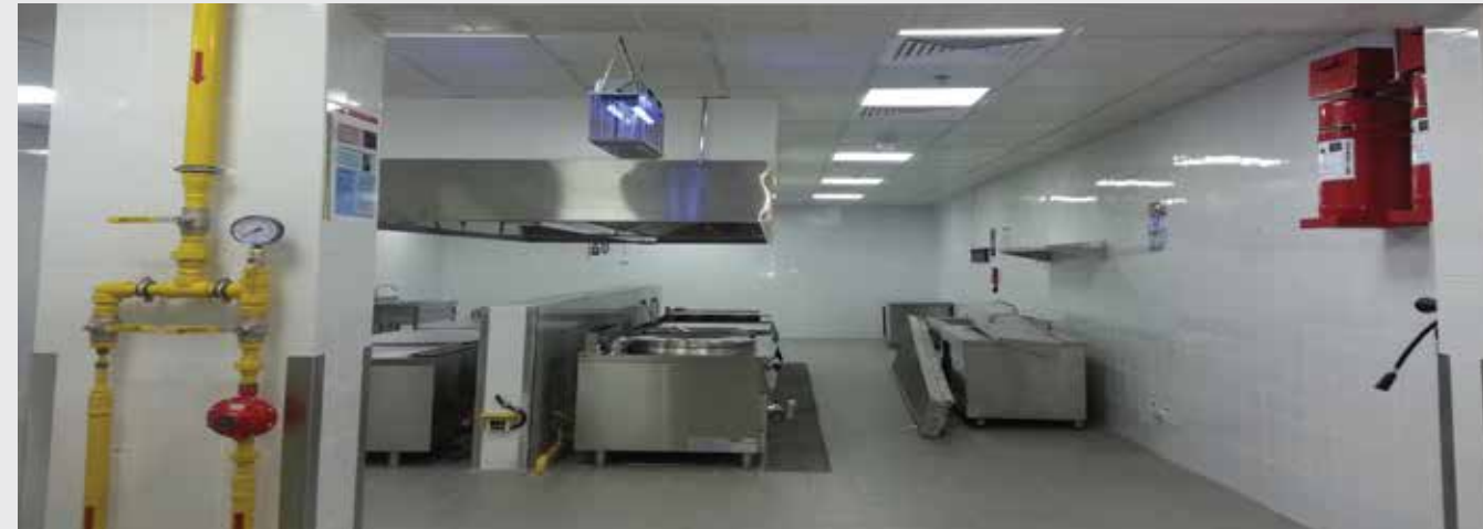
CENTRAL KITCHEN - KELVIN CATERING SERVICES LLC. ABUDHABI.
